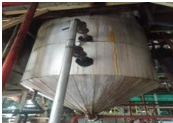
Gambar 2. Continuous settling tank.
