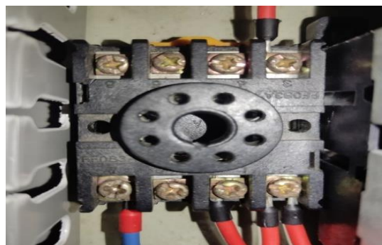
Gambar 7. Instalasi Time Delay Relay
