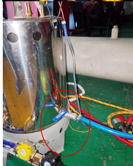
11 Emergency water draining valve
