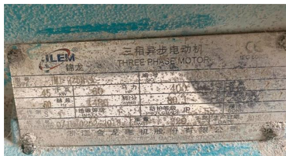
Gambar 5. Nameplate Motor Listrik Water Jet Pump
